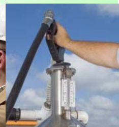
Fuel pump calibration
